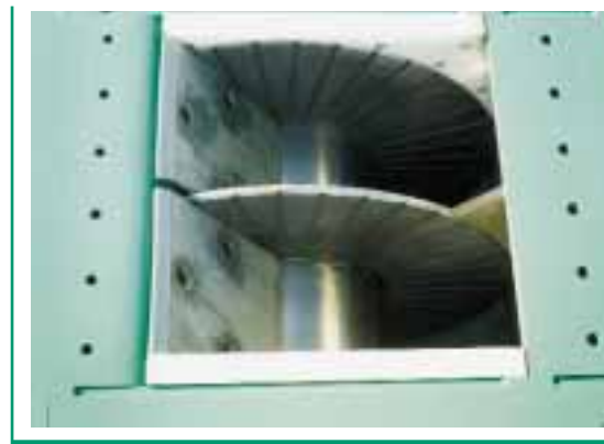
Internal view of two-duct feeder
