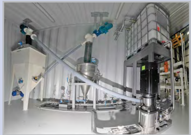
Water treatment system inside an ISO container
