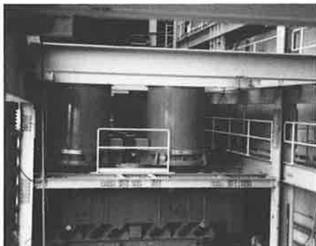
An installed Boiler Feed Train
