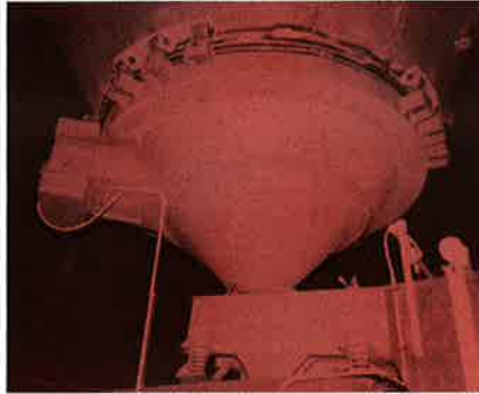
Fig. 18: Bin Activators usually are not readily accessible for maintenance.
