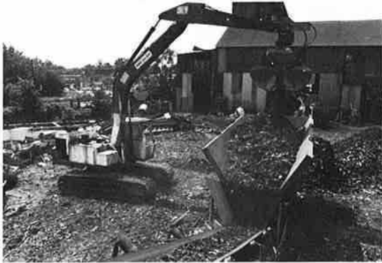
Abusive crane bucket loading is routine
